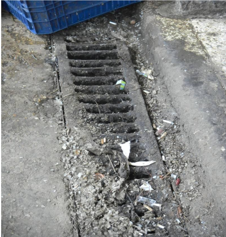
Photo 5: Moneab retail market gutter, Cairo
