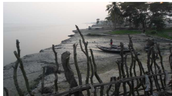
Fig. 5. Photographic view of bandaling structure used for controlling bank erosion at Kajal river side in Galacipa
