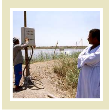
Electricity has now been installed on Nazmy Abdel Rabman's fish farm. Investing some of the farm's profits in this way will allow Nazmy Rabman to better control the water quality of his ponds, so increasing his farm's productivity.
