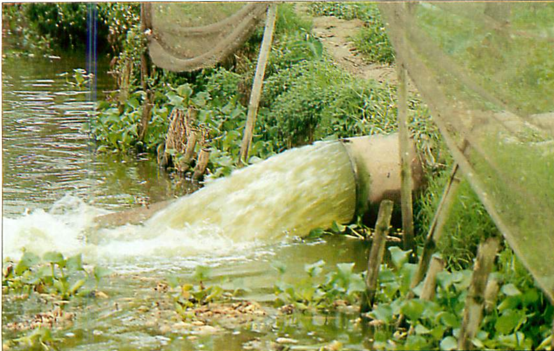
Wastewater after treatment in fishponds.
