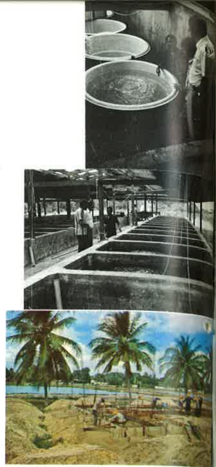
Top: Algae production tanks, Prachuap Khirikhan station. Center: Multipurpose rectangular tanks. Bottom: New pond construction, with large holding ponds behind, Prachuap Khirikhan station.
