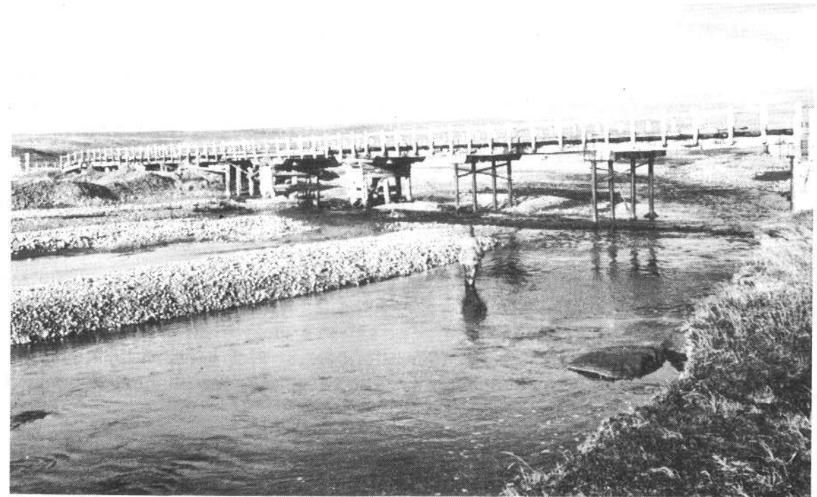
Figure 28. Brunswick Peninsula; Rio Grande bridge. Note repairs.
