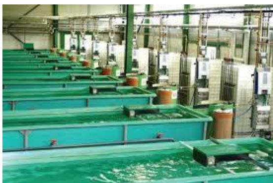
Plate 14: Re-Circulatory System Facility
