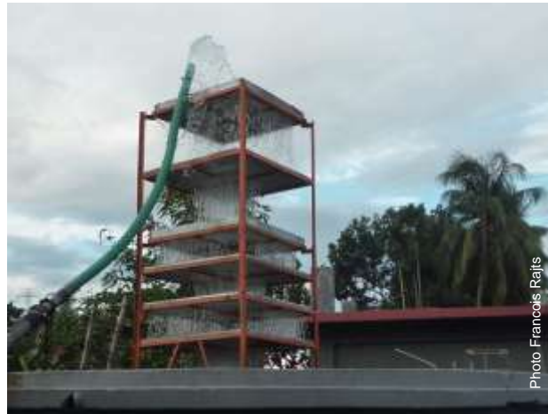
Plate 7. Water aeration structure (water tower) in Bangladesh.
