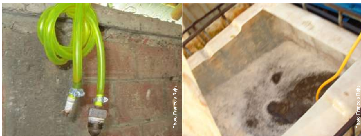
A locally made adapter to a cylinder, without a manometer, called a budka . This is a bad practice, because it supplies only one tank/diffuser.
