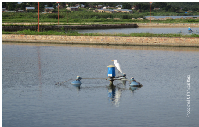
Plate 5. Vertical pump aerator is practical for standby emergency operations too.
