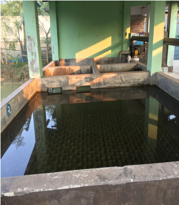
Water Recirculation Plant (partial view)
