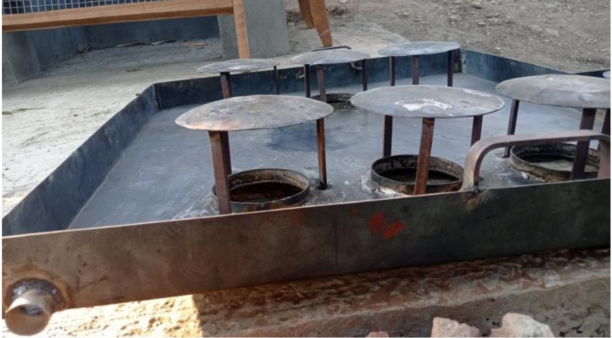
Figure 33: Well-fixed coned shaped caps
