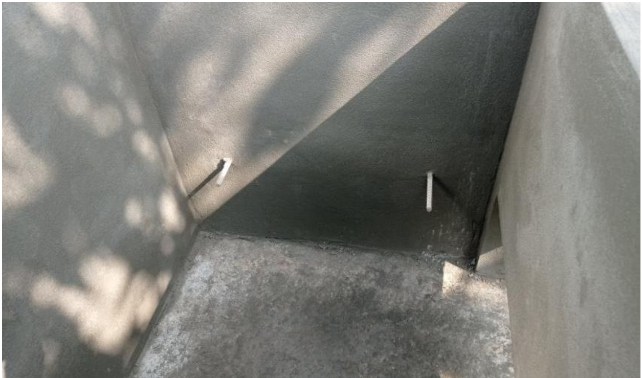
Figure 10: Place 4 pieces of rebar on the sides of the kiln wall to hold the fat collection tray in position inside the kiln chamber
