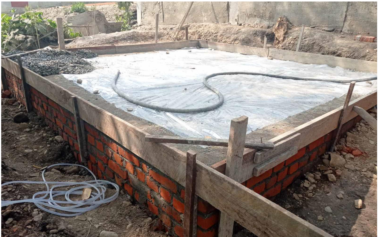
Figure 4: Laying a 3-inch thick reinforced concrete base as the base for the kiln
