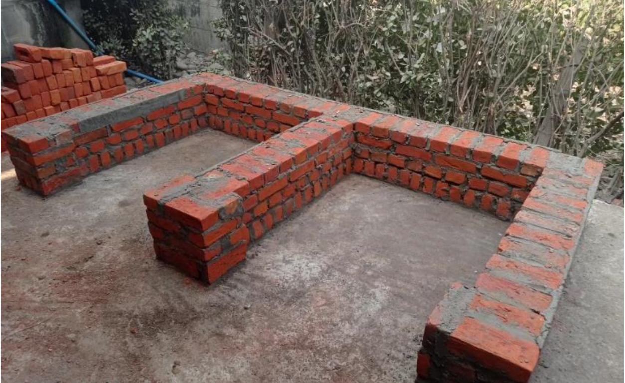
Figure 5: Precise brick work according to the measurements is important from the beginning
