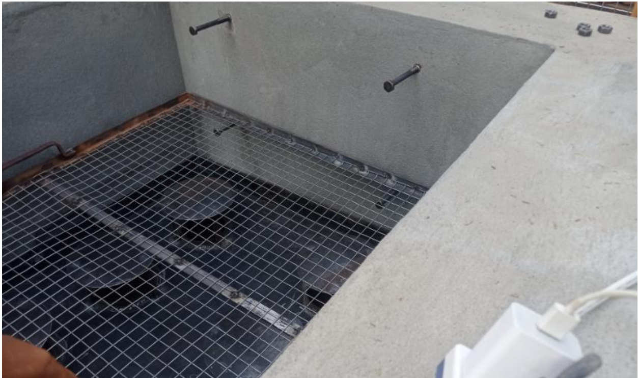
Figure 14: Fat collection tray under the smoking rack inside the kiln chamber
