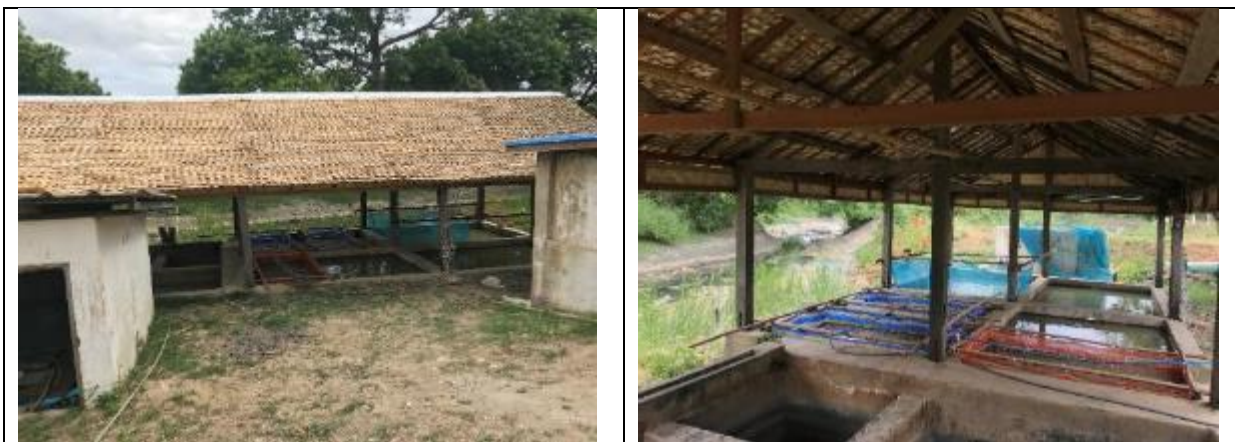
Photos 01 and 02. The renovated and extended roof over external concrete tanks at the DoF Nad Yay Kan hatchery which has been used for nursing and sex-reversal of GIFT seed.
