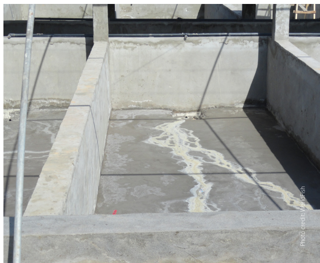
Plate 1. Traditional concrete tank for tilapia spawning.
