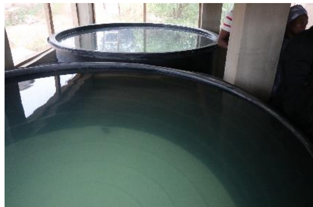
5000ltrs tank filled with water and soda ash to regulate PH
