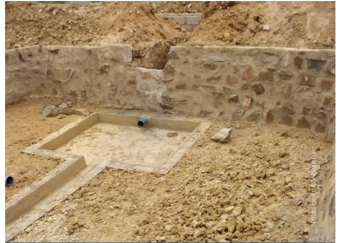
Plate 2. Construction of a concrete catchment at the lower end of an earthen pond.
