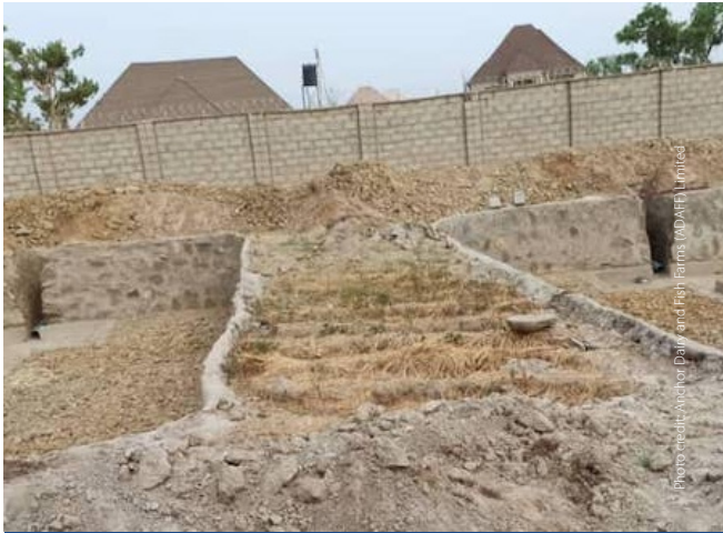
Plate 1. Construction of a concrete catchment at the lower end of an earthen pond.
