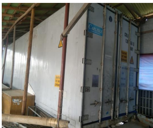
Fig 51: Cold storage (Freezer)
