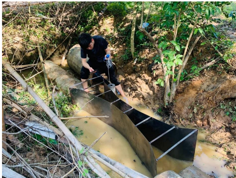
Figure 5: Parshall Flume and water level sensor installation at the outlet of the fish pond
