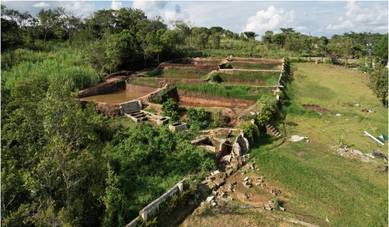
Damaged pond walls and tanks resulting in fish escaping
