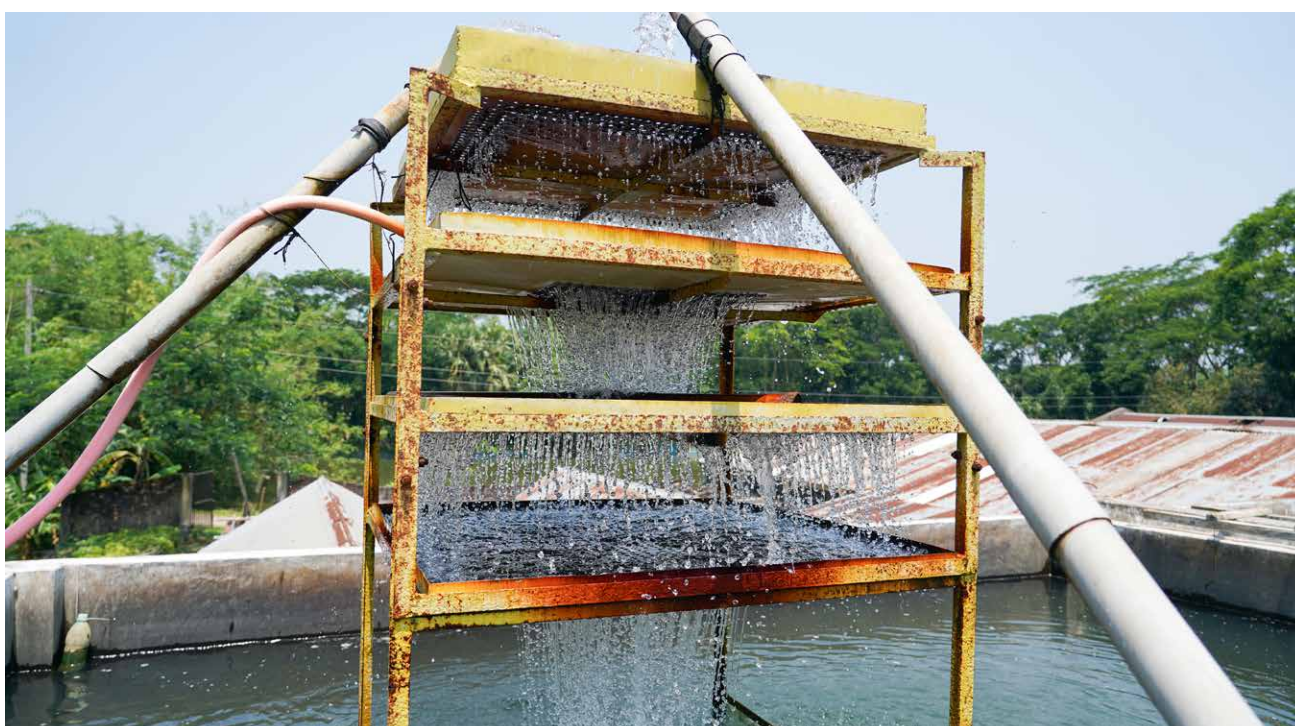
Photo 10. An aeration tower in an overhead water reservoir tank at a hatchery. Photo credit: Harun Or Rashid, WorldFish.
