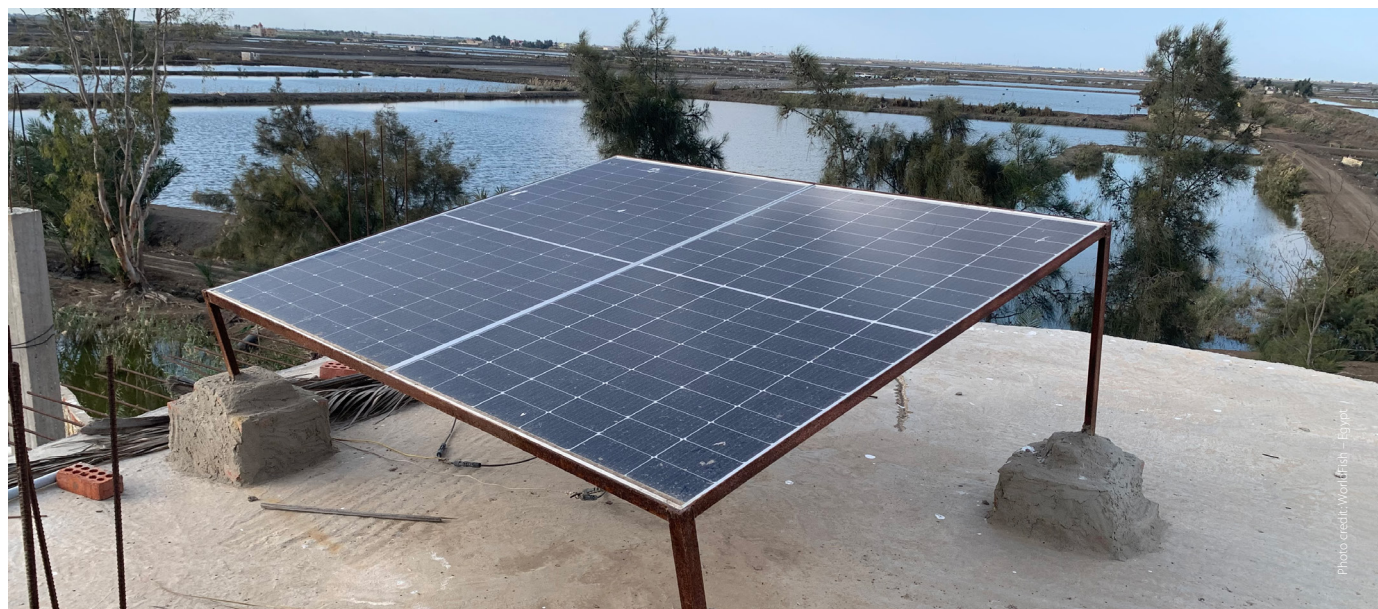
Figure 7. Solar PV panels installed at a fish farm for energy supply and lighting.
