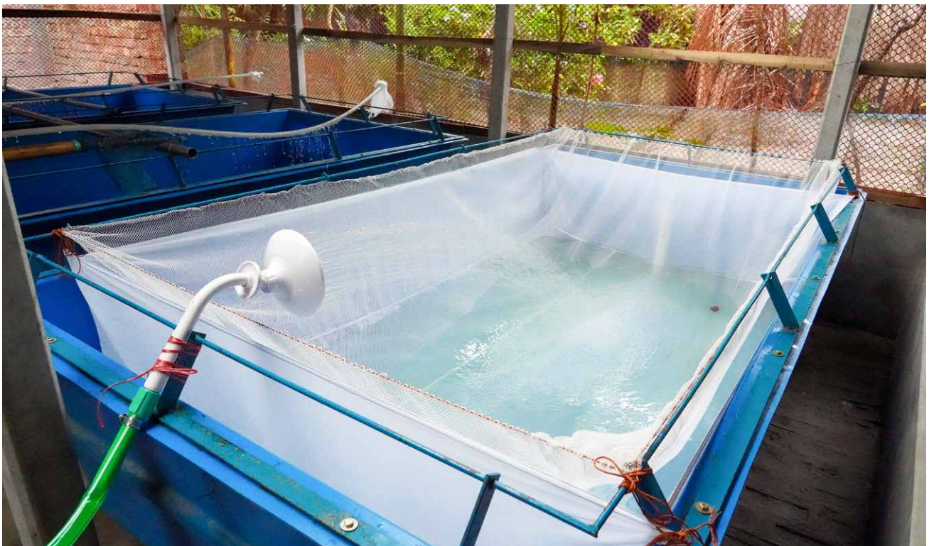
Photo 7. Installation of inner and outer hapas in an FRP tank. Photo credit: Dr. Hazrat Ali, WorldFish.
