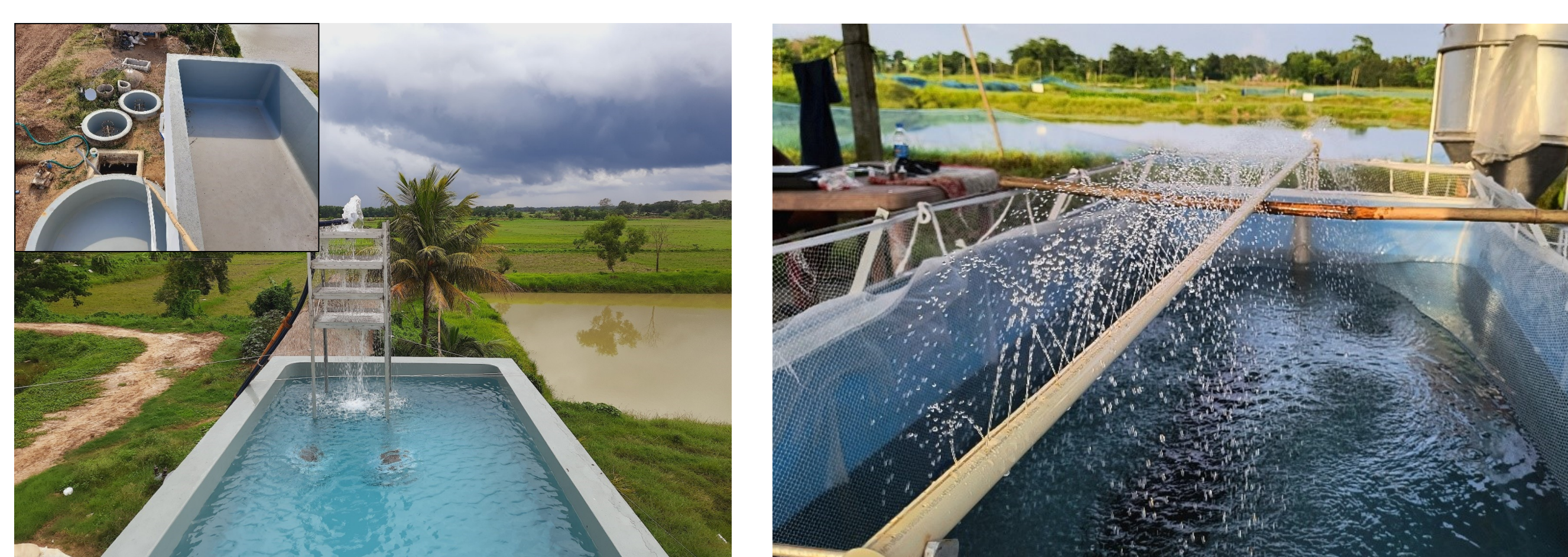
Aeration tower installed in overhead water reservoir tank for constant showering of oxygen-rich water
